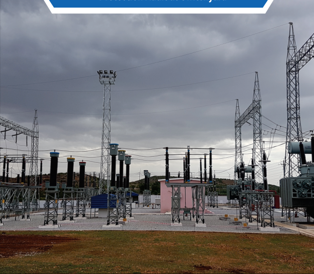
Protection Audit at Switchyard
