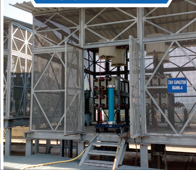
Switching Surge Measurement at Capacitor Bank
