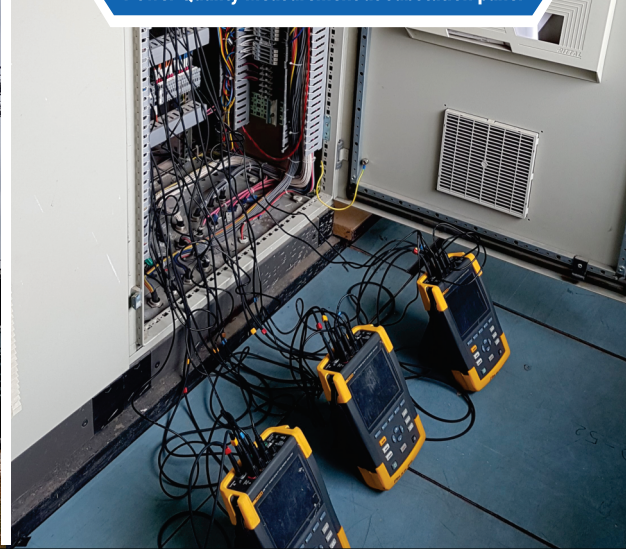
Power Quality Measurement at substation panel
