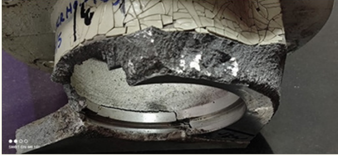
Figure 1.2.6 (a): Photograph of failed aluminium flange of transformer bushing
