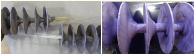
Figure 1.2.5(a): Failed polymer insulator (left) and section of insulator showing silicone sheath with degradation and cracks (right)
