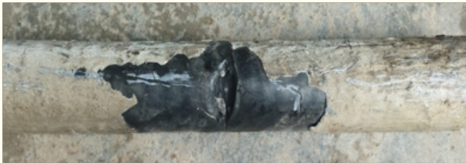
Figure 2.2.1(a): Failed 132 kV cable
