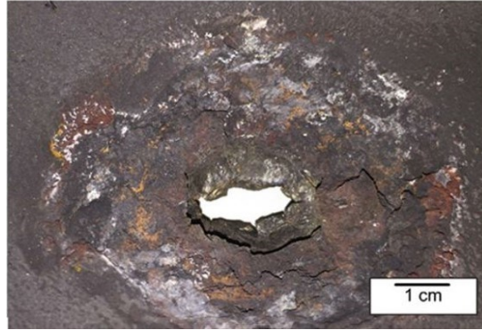
Figure 9. Caustic corrosion failure of tube. It shows white color deposits near the rupture [9]
