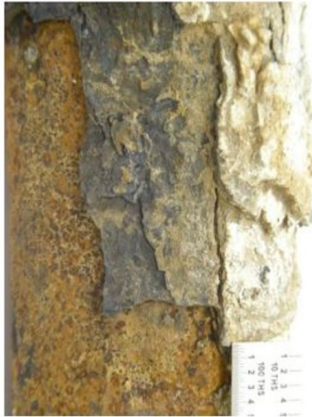
Figure 7. Photograph of superheater tube surface with thick deposits due to corrosion [5]
