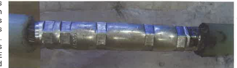
Figure 3: Failed part of the 66-kV cable joint.
