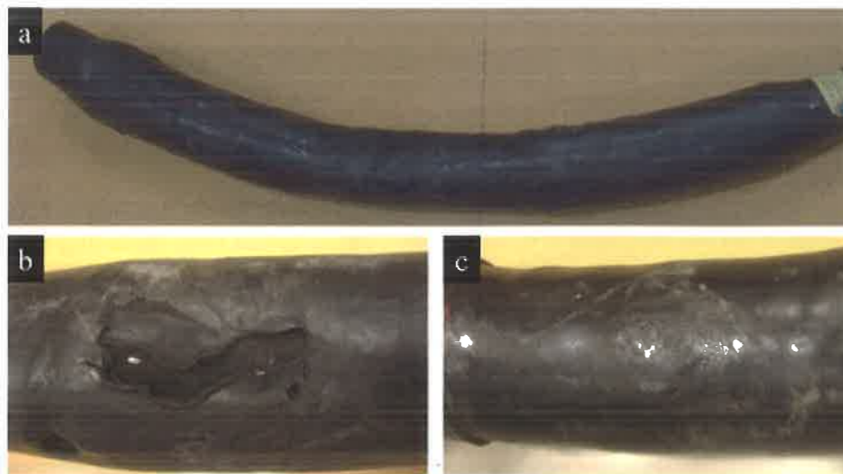
Figure 1: a) Failed 33 kV cable joint, b) Puncture on the joint, c) Outer sheath showing indications of overheating.
