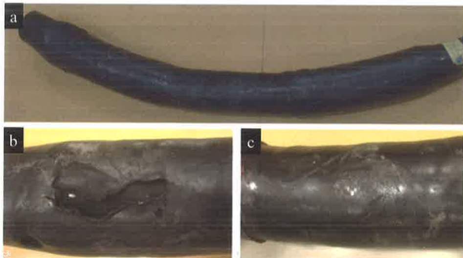
Figure 1: a) Failed 33 kV cable joint, b) Puncture on the joint, c) Outer sheath showing indications of overheating.
