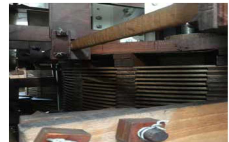
Figure 2: Crack observed on End press ring of Y-phase winding due to heavy pressure
