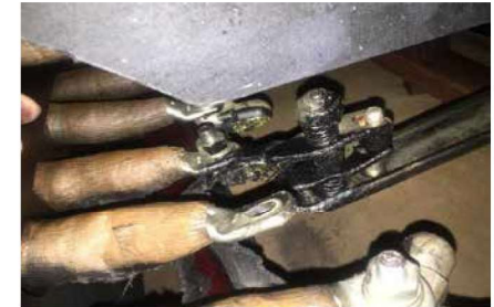
Figure1: Melted contacts resulting in a joint (weld) at one position of R-phase tap changer
